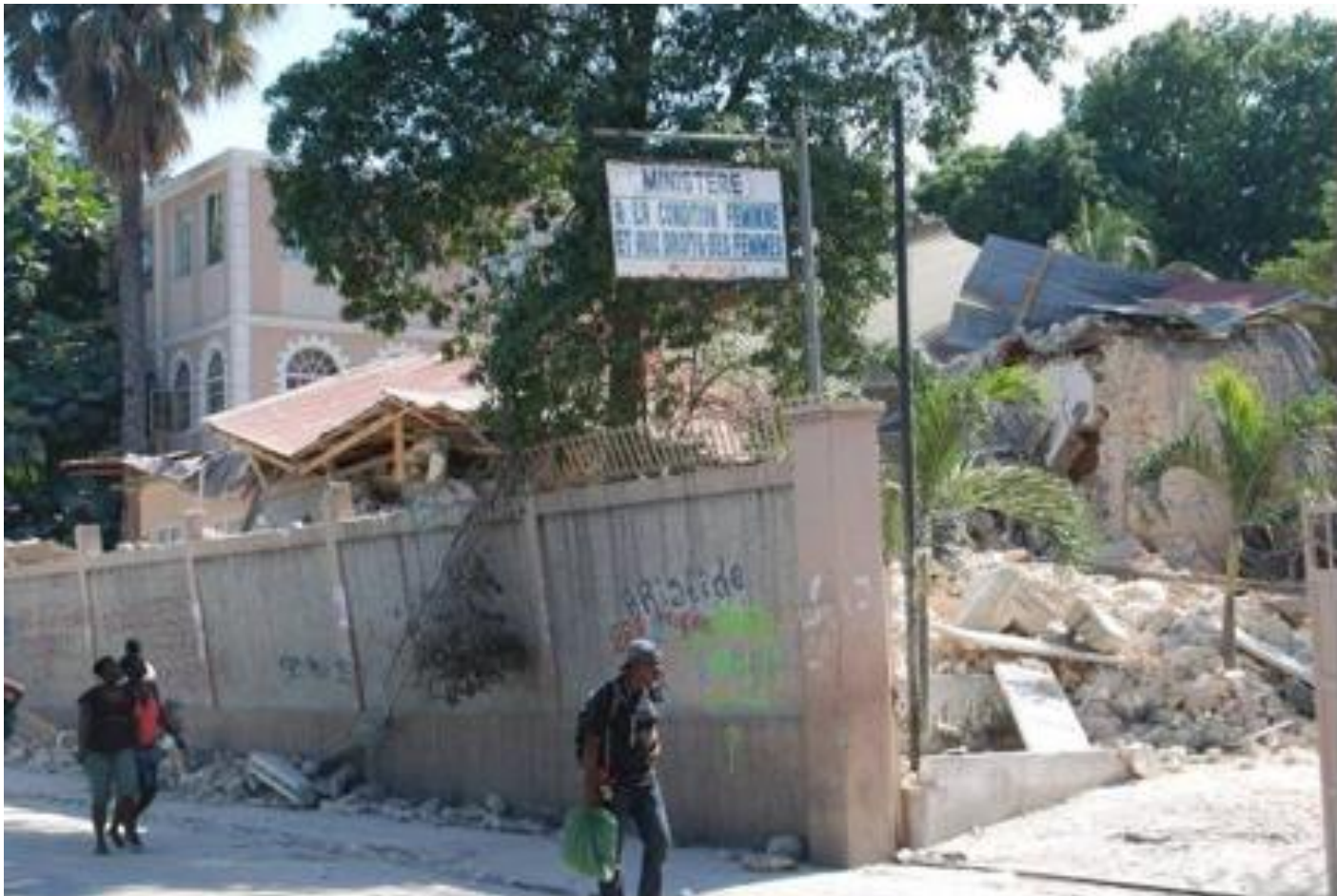
Government buildings, like the Ministry of Women's Affairs, suffered severe damage rendering them unusable. Photo credit OTI/HAITI Ops Damage Report.
